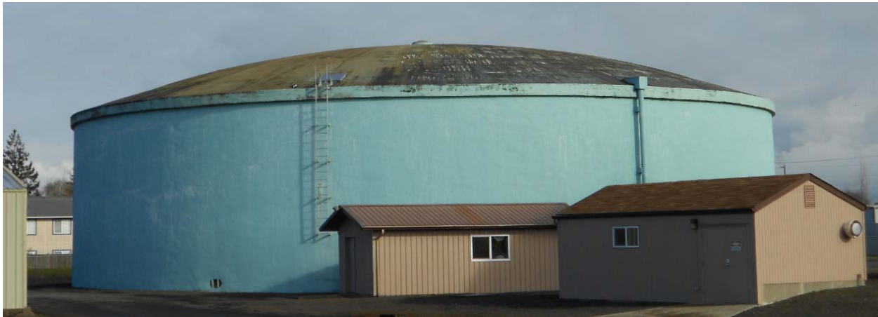
City's 2-Million Gallon Water Storage Tank
